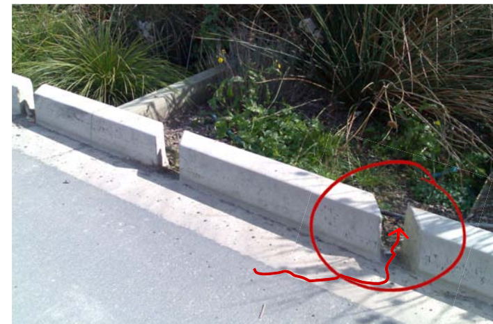
Incorporate on-site landscaping with storm water management. This example captures runoff from parking areas, channelling it to a rain garden via kerb cuts to filters before discharging to the piped system.
