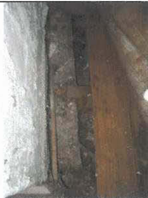
Rotten floor joists in hallway
