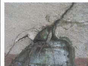
Deterioration of plaster, mortar joints and brickwork due to vegetation growth at base of walls
