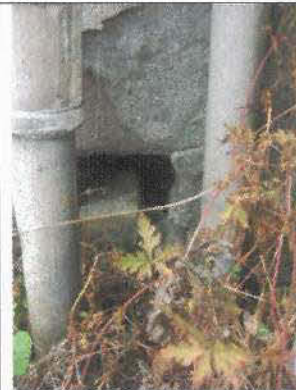
Missing bricks at base of north west corner
