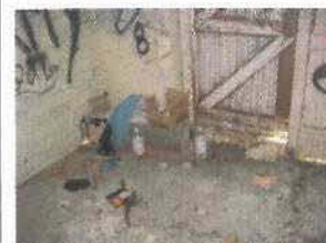
Occupation of derelict building by homeless
