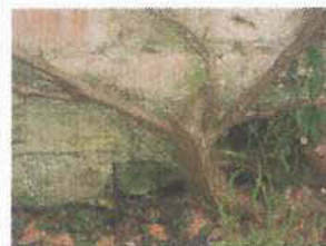
Extensive growth at base of brick wall east façade, root work damaging shallow foundations
