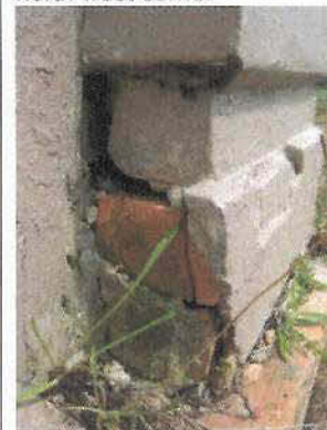
Cracking and spalling of brickwork at base of north west corner
