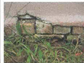
Missing plaster and mortar joints at base of brickwork north west corner
