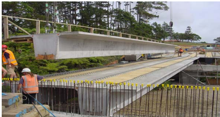
'Bridging the Gap' from Summerland Drive, in Western Heights to Munro Road Ranui
