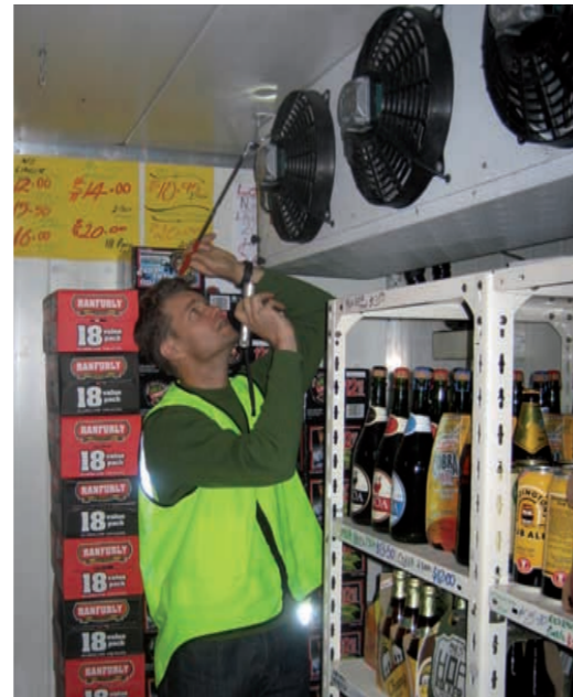
Ecomatters Energy Efficiency Advisor Bell Bell inspects a refrigeration unit
