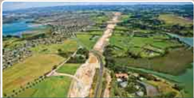
The path of the motorway can now be clearly seen on the landscape
