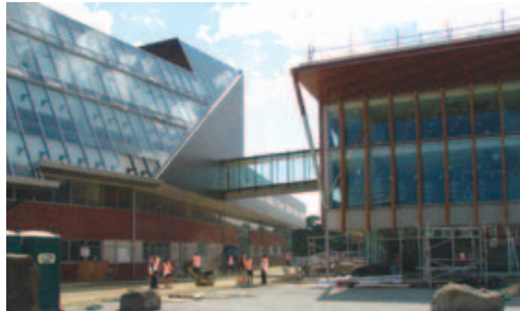
The new Waitakere Central Library, in Henderson, is designed to give the highest level of access to information demanded by a modern city, its businesses and a rapidly expanding tertiary sector.
