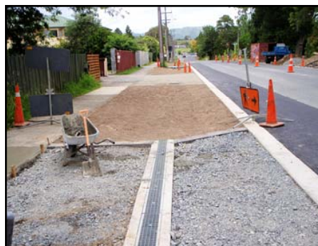
Providing road widening for improved safety and swale drains for sustainable water quality collection
