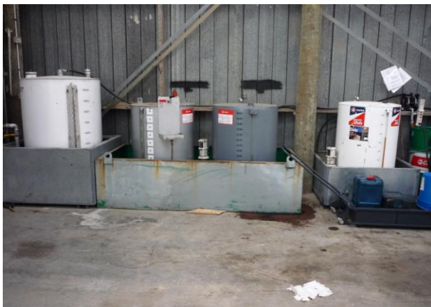
Bunded engine oil tanks in the fleet servicing workshop.
